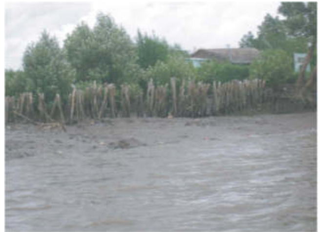
Fig. 5. A typical timber piling constructed by residents, combined with vegetation for protecting river bank from ship waves in Kinh Sang River.
